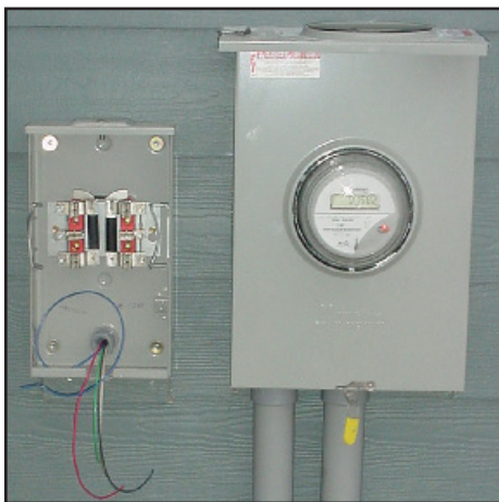
CT Sub Meter box with appropriate wiring.
